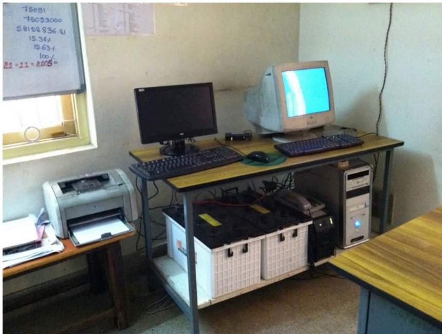
Computers with spare batteries
